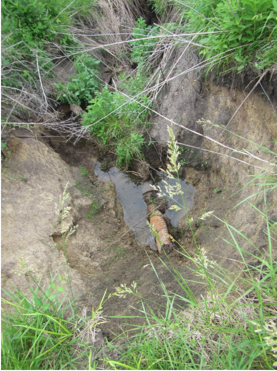
Broken outlet pipe of pond 221, and resulting gully.
