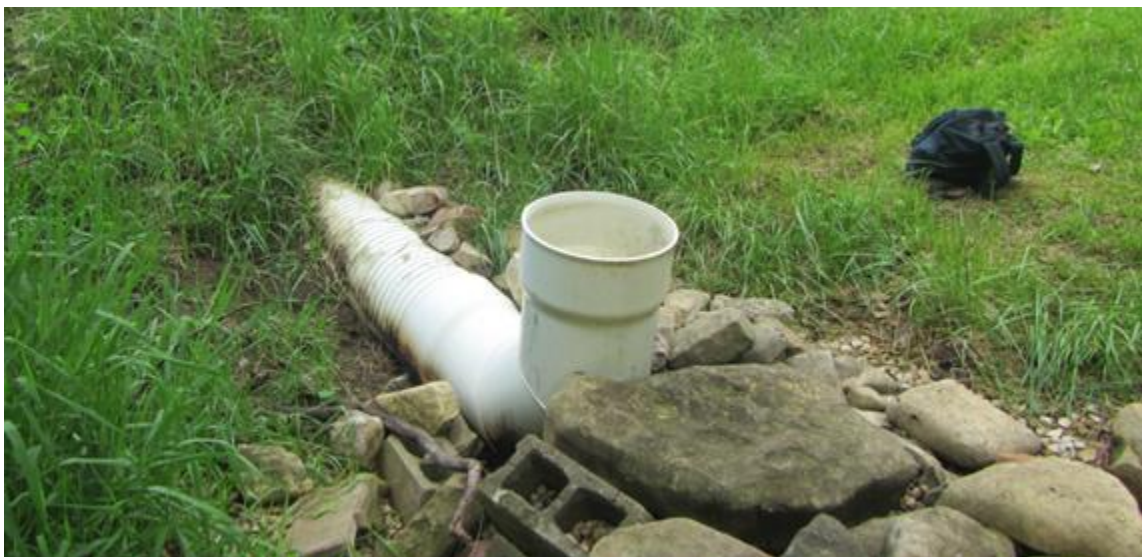
Figure 20. Pond 183 standpipe, the underside of which is cracked allowing water to pass. Also note the lack of a trash guard that would reduce debris from plugging the outlet.
