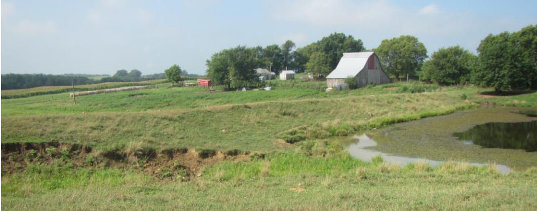
Figure 19. At pond 262, the eroded spillway is seen in the left foreground.
