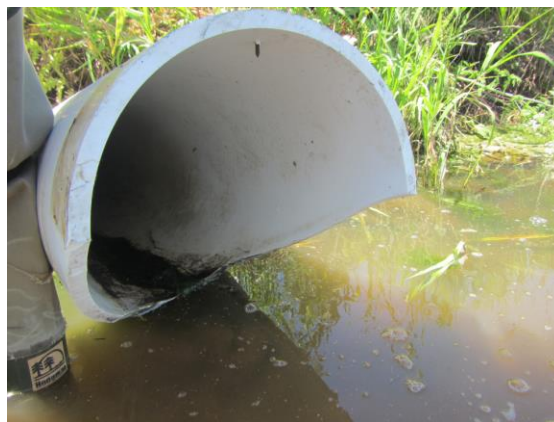
Figure 16. A beveled cut in the stand pipe opening may have been the landowner's attempt to reduce debris buildup on stand pipe at pond 279. The opening of the 30 cm diameter pipe was 2 mm above the surface of the water.
