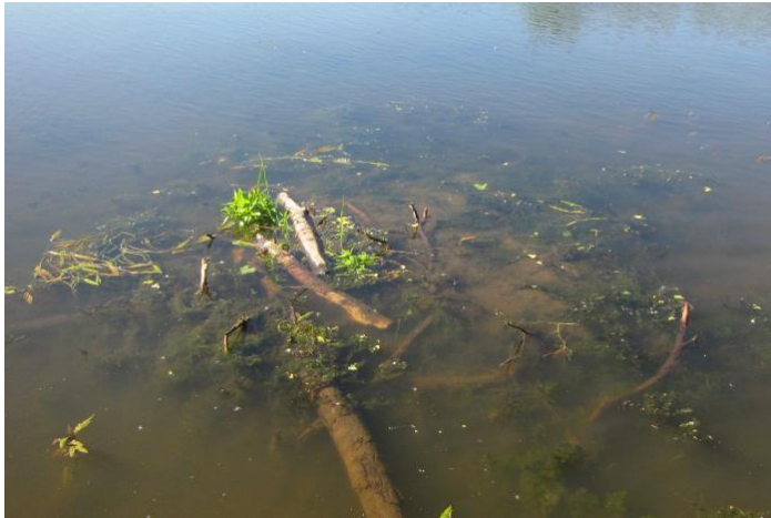
We were not able to locate the stand pipe at pond 223. This might be it, blocked by beavers and sediment.
