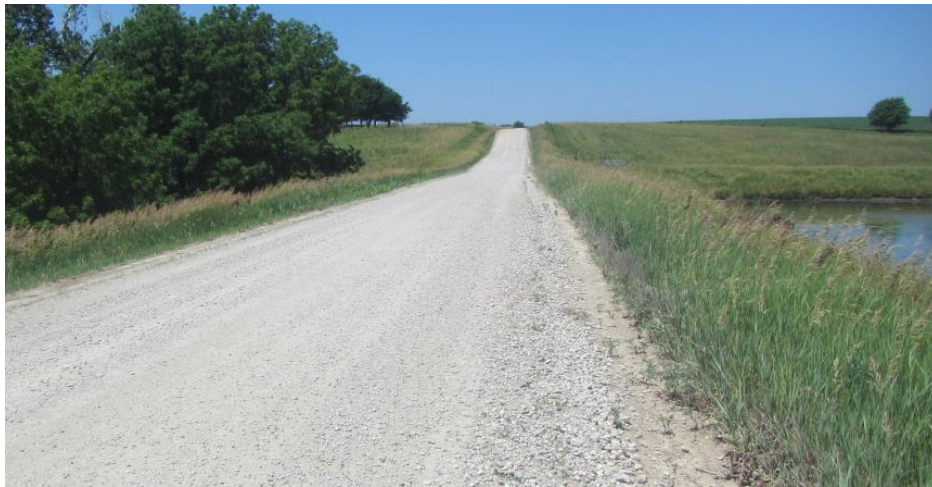
Figure 13. Few dams also function as a road such as pond 172 (high point elevation 2.505 m above water level, 0.635 above spillway low point).
